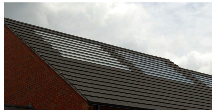
▲ Solar panels are integrated into the roof in Upton. Benefits include, aesthetics, maintenance, safety, and pest control.
